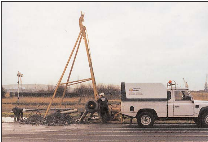
Construction of a borehole for the installation of groundwater monitoring and sampling standpipes
