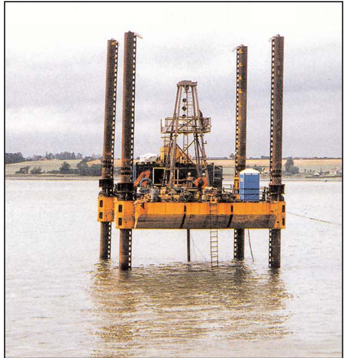
Cable percussion boring and large diameter wireline coring from a jack-up platform
