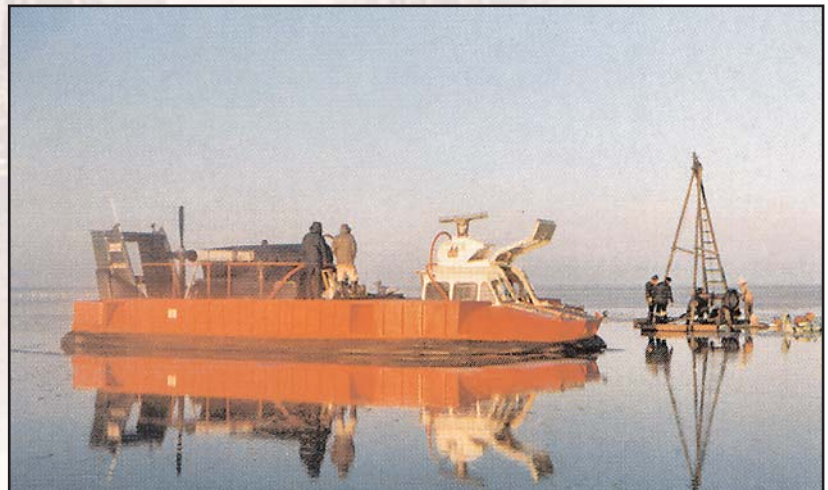
Investigation on tidal mud flats using a cable percussion rig transported between exploratory locations by a hover freighter
