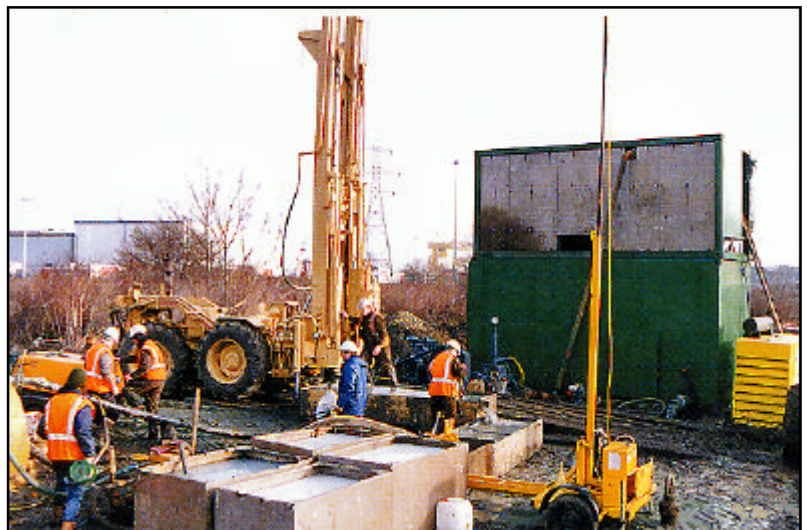
Construction of a large diameter pumping well using a polymer based recirculating system
